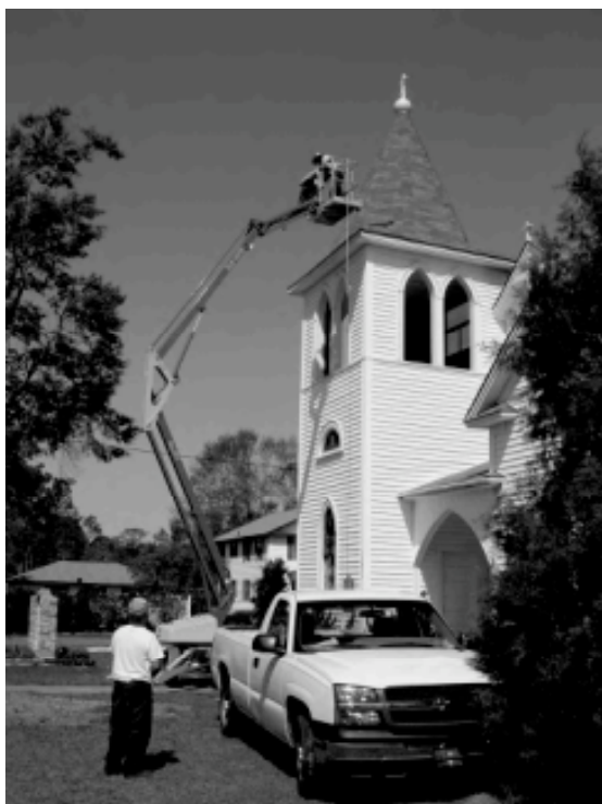
Figure 12. In 2005 President Peter Midgarden (on the left) and Ralph Utter worked to repair the steeple shingles after Hurricane Ivan. The steeple was constructed with the church in 1915-1916.
